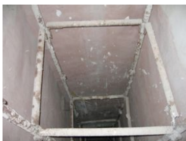
The Lift Shaft – sadly still in the same condition!
